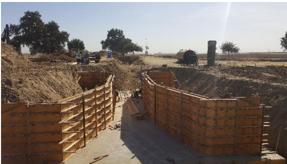
Installation of new contracted weir for SCADA Phase II Grant. (Phase 1 Construction)
