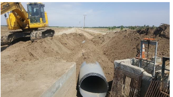
Replacing existing metal culvert on Kaweah Ditch with new 48in. HDPE pipe.
