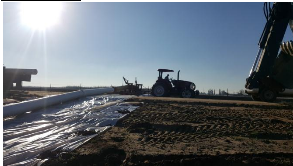
PTO pumps at Swall Basin.
