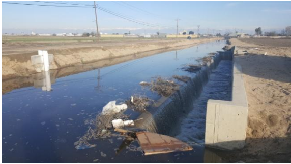
Trash at Oakland Colony long-crested weir.
