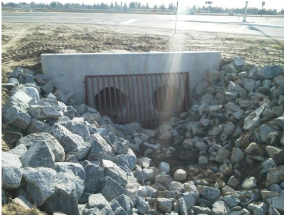
New trash racks on Liberty Ditch.
