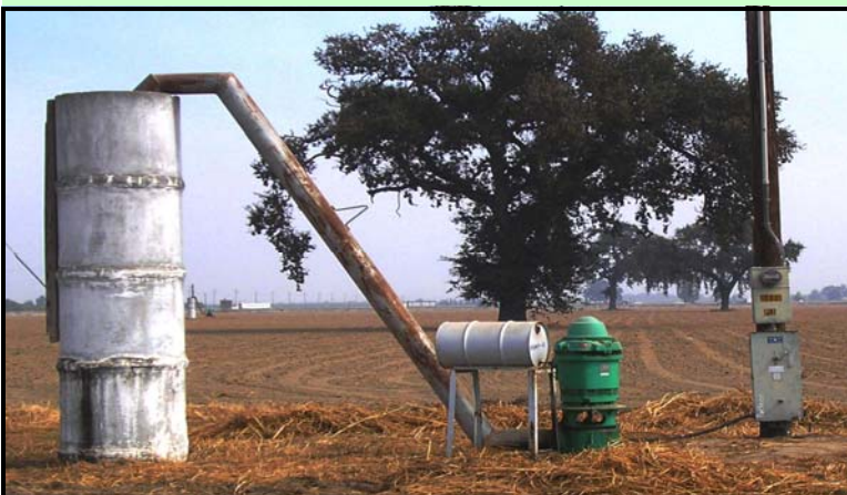
Local Private Groundwater Well
